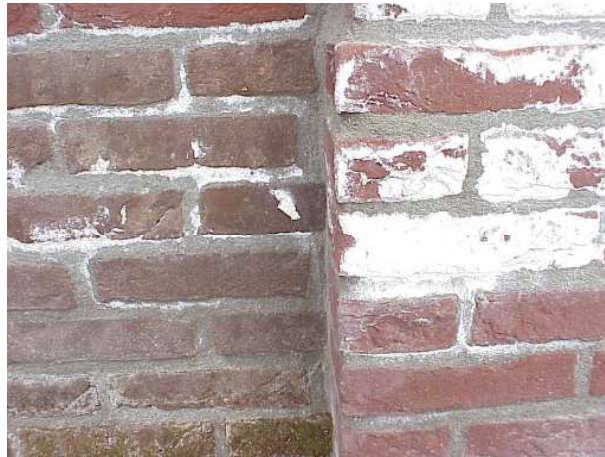
Figure 1.1: A typical example of salt efflorescence.
