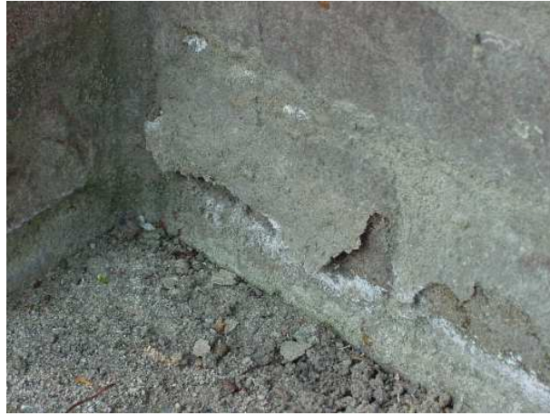
Figure 1.3: Lower part of the wall of figure 1.1 after four years: a layer of material is chipping off.
