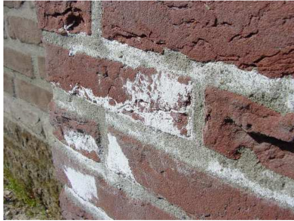
Figure 1.2: The same wall as in figure 1.1 four years later. It can be seen that the efflorescence has decreased but the lower part of the wall is covered with moss.
